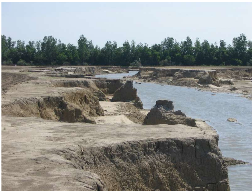
Figure PD11. A 3 m deep, 25 m wide, and 700 m long gully created by the water rushing through the made-induced Birds Point levee breach. Reprinted with copyright permission of the Editor of the Open Journal of Soil Science.
