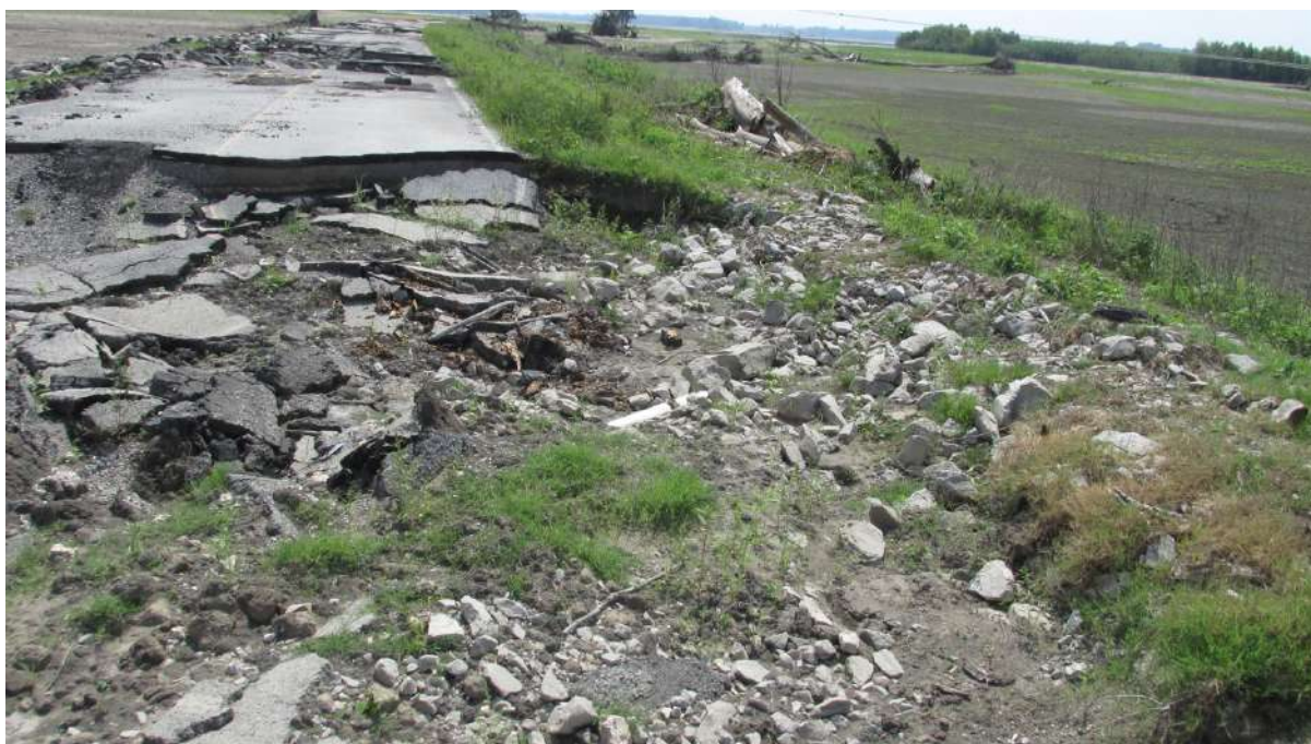
Figure PD16. The roadbed of an Alexander country highway was destroyed by flowing water through a breach in the Len Small levee. Photo Credit: Lois Wright Morton. Reprinted with copyright permission of the Editor of the Open Journal of Soil Science.
