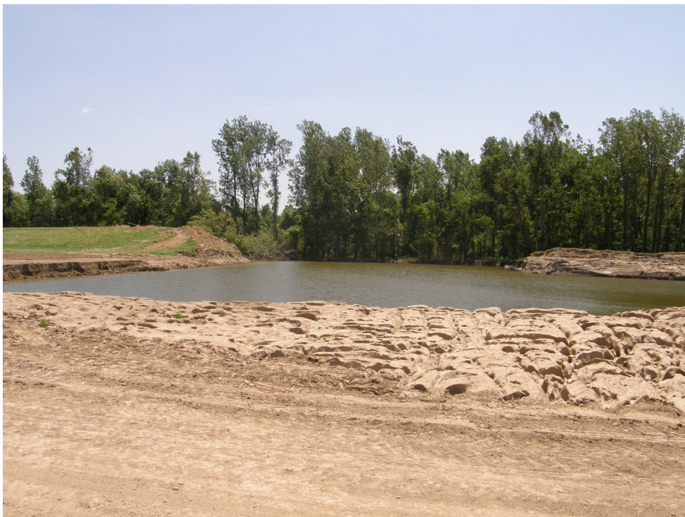
Figure 3. The first of three Birds Point levee breaches was triggered using TNT by the U.S. Army Corps of Engineers. The crater lake is between the levee and the adjacent farmland. Photo credit: Kenneth Olson. Reprinted with copyright permission of the Editor of the Open Journal of Soil Science.
