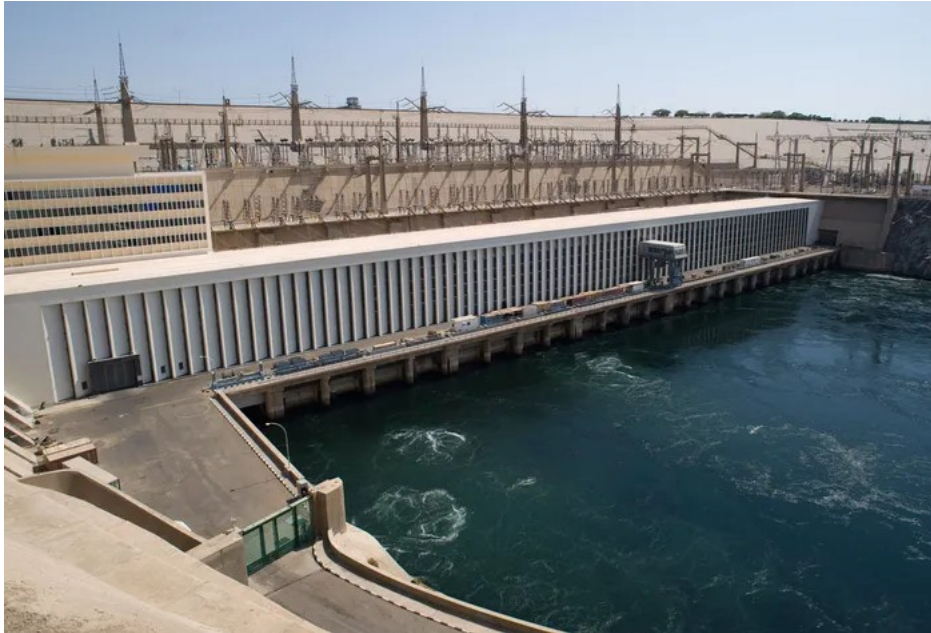
Figure 2. Power pylons at the power plant of the Aswan High Dam. Photo credit: Vyacheslav Argenberg. Reprinted with copyright permission of the Managing Editor of the Open Journal of Soil Science.
